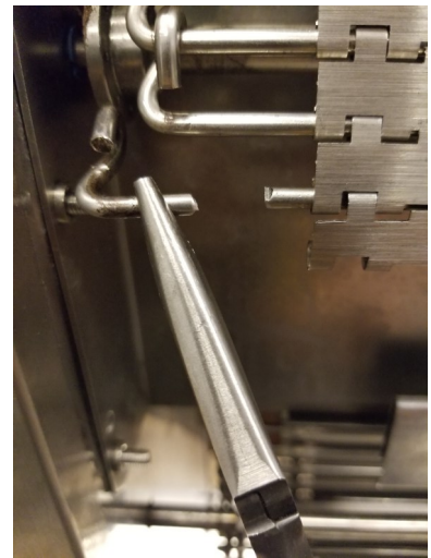
View of the cut wire
