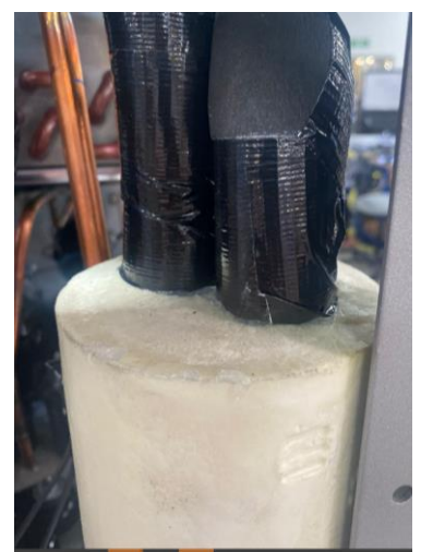
Closed cell insulation covers copper and firmly contacts the factory foam. All seams in tubing insulation are sealed with duct tape.
