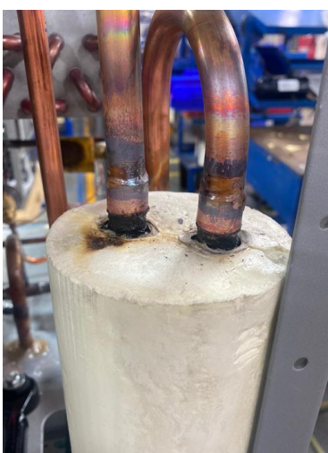
Factory foam shows damage after brazing.
